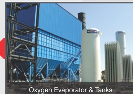
Oxygen Evaporator & Tanks
