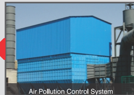
Air Pollution Control System
